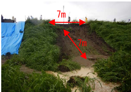
崩落箇所②
