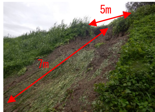
崩落箇所③
